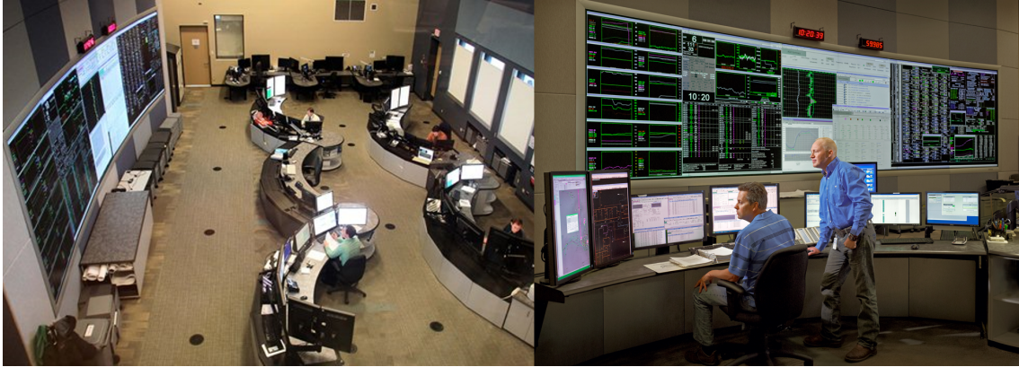
Figure 5.1: Pictures of the current control room in AESO Control Centre. 7
